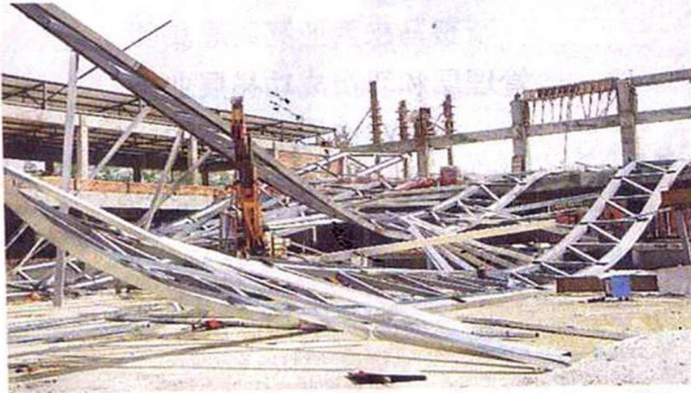
FALLEN ROOF: Indonesian worker Sumaidi was killed when the steel roof structure of the bowling stadium collapsed in Paroi, Negri Sembilan, yesterday.
