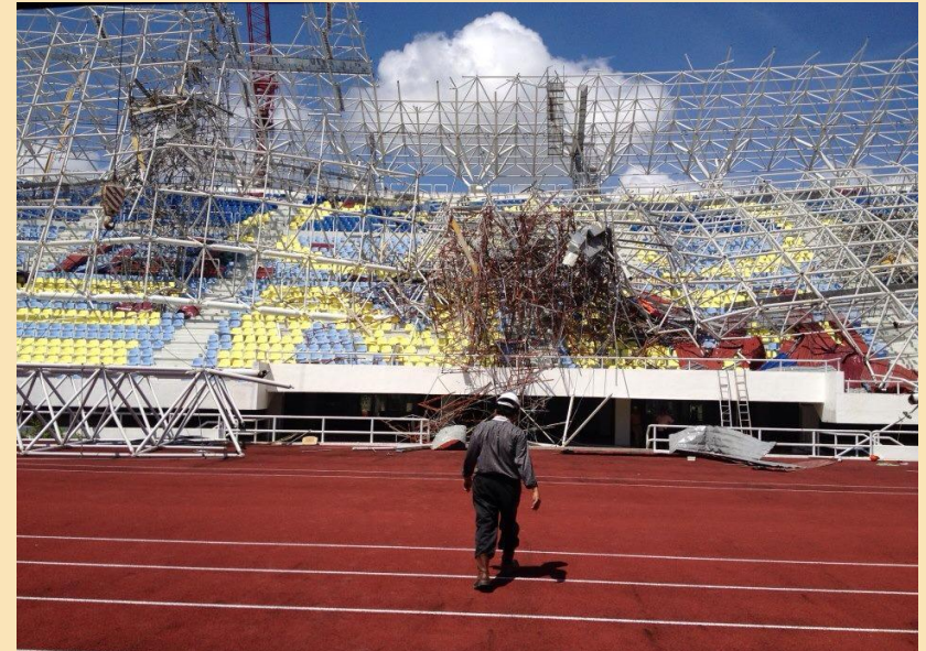
Collapse of the scaffolding of repair work on the same stadium in 2013, February 20 th , 11.30am. Two workers injured (broken legs).
