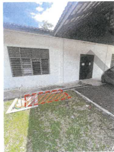
LOKASI ASAL EMERGENCY SHOWER
